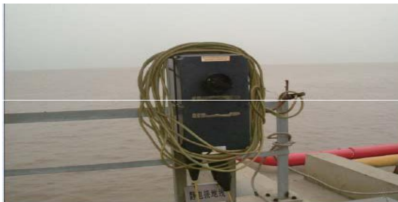
Figure 8.9.3a Bonding cable installations on shore
