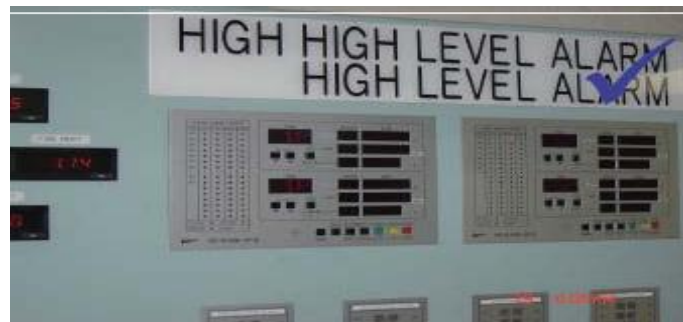
Figure 8.12.2a Alarm panel for high level and high high level in cargo control room
