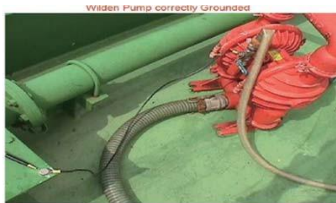
Figure 5.2.7 Portable pump and bonding arrangement
