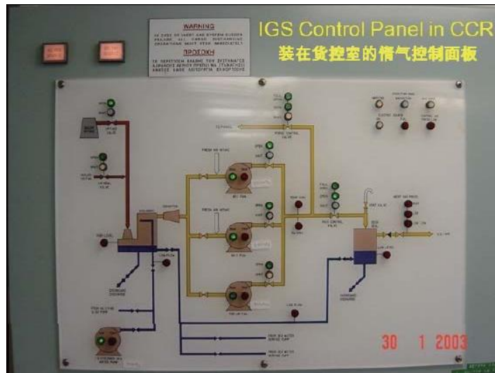
Figure 8.12.2c Control panel for inert gas system in cargo control room
