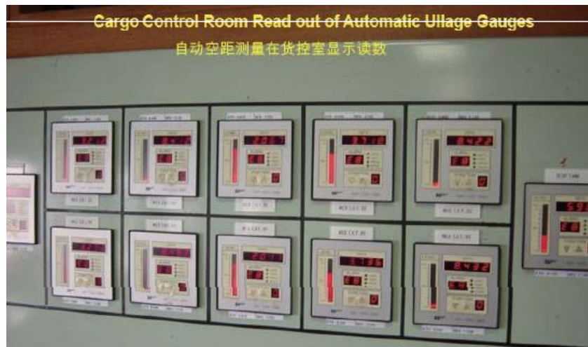
Figure 8.12.2d High level indicators in cargo control room
