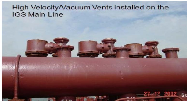
Figure 7.1.4c High velocity/vacuum vents installed on the IGS main line
