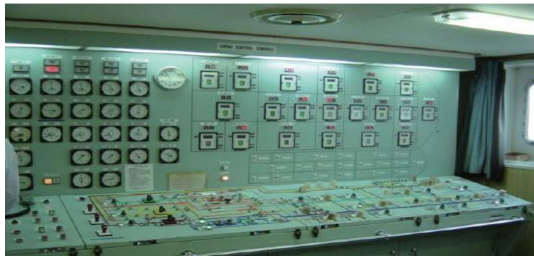
Figure 8.12.1 Control panel for cargo and ballast operations in cargo control room
