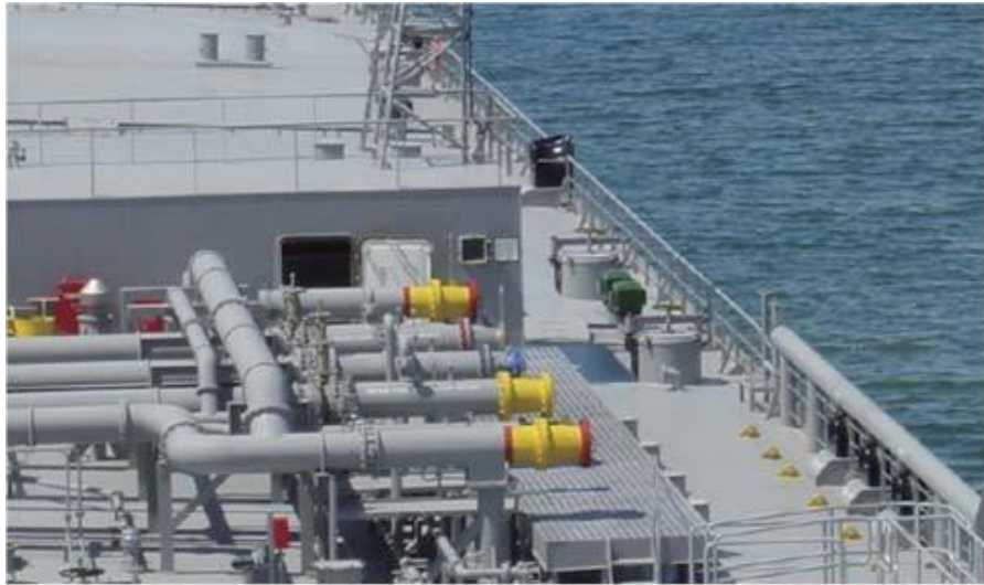
Figure 3.3.11 Hose supports in way of the ship's side abreast of the manifolds
