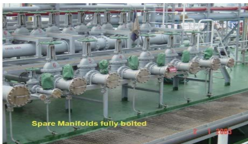
Figure 8.2.7 Spare manifolds fully bolted on the deck
