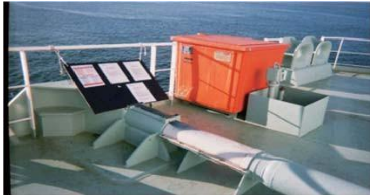
Figure 5.2.9 Spill tank of enclosing of the vent pipes (air pipes) of tanks containing flammable fluids
