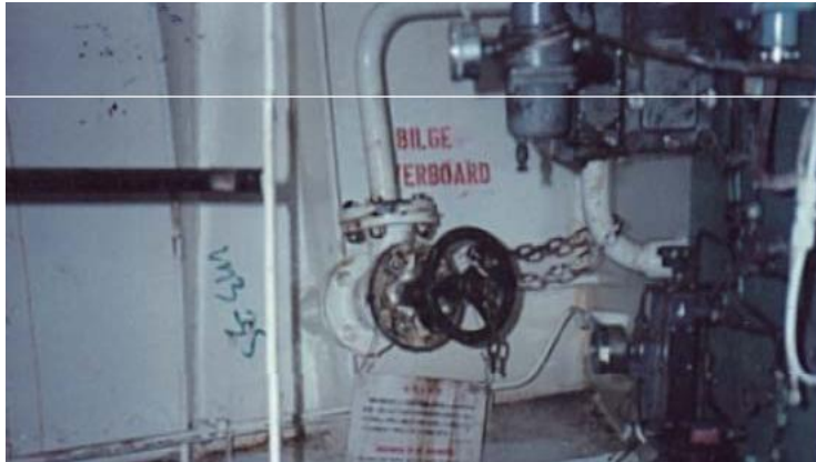
Figure 5.6.11b Overboard valve of oily water separator in engine room closed and sealed when in port
