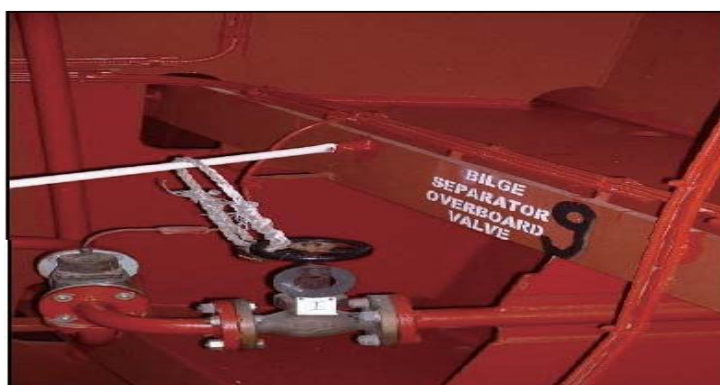
Figure 5.6.11a Oily water separator discharge valve in engine room closed and locked when in port
